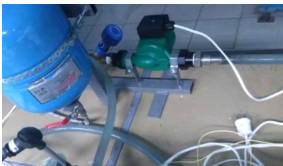
Figure 5.4 – The part of the appearance of the experimental installation
